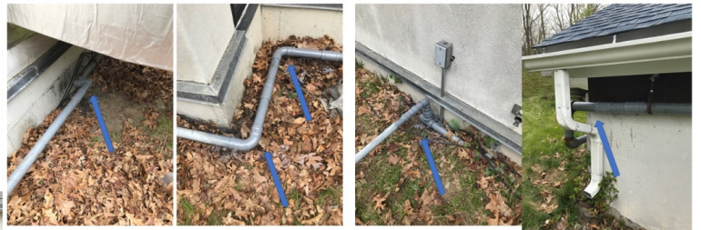
The spot leaked the most
